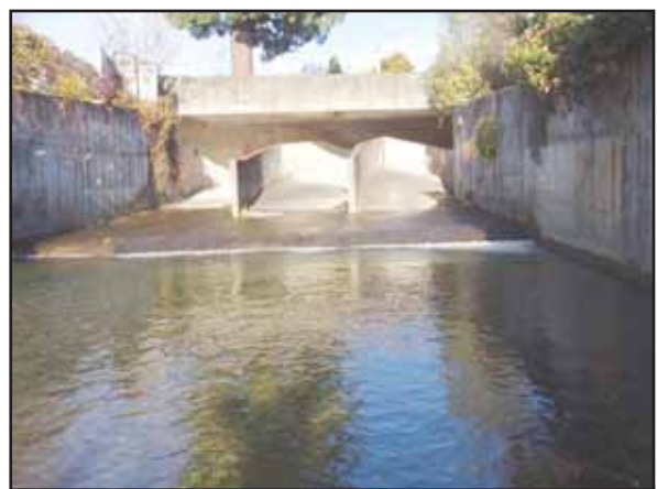
The culvert at Nile Street presents a barrier for native fish migrating up the Brook
