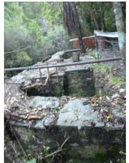
Historic structures from the 1868 waterworks after being cleared by members of the track cutter team.
